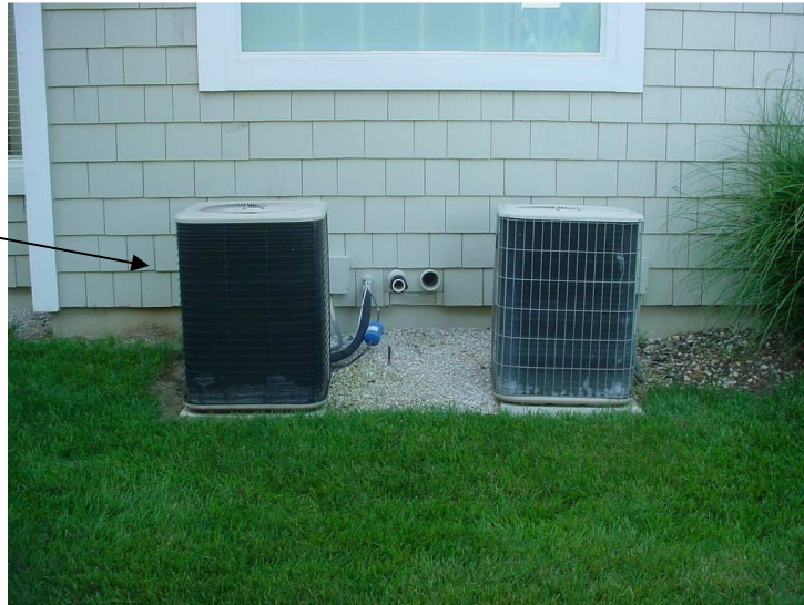
The arrow is indicating the newer of the two units
